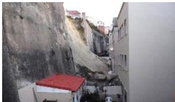
Figure 2. View of earth retaining walls after its partial collapse
