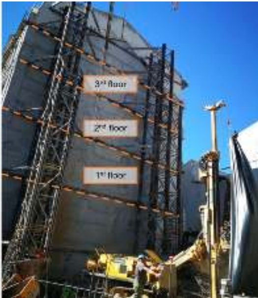
Figure 6 – Current phase of the site works: facade retention of the neighbour building and demolition (March 2019)
