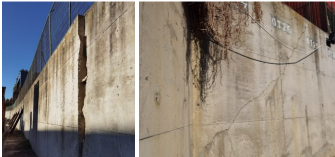
Retaining walls pathologies
