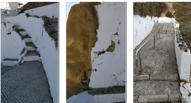
Figure 2. Staircase structural pathologies.
