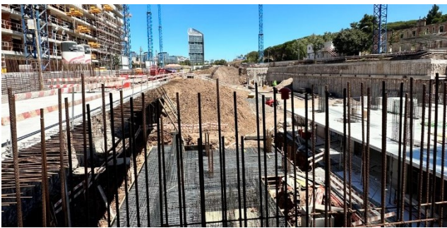
Figure 14 - West Side (Left) and East Side (Right) solution at bottom excavation. (definitive structure already in place).
