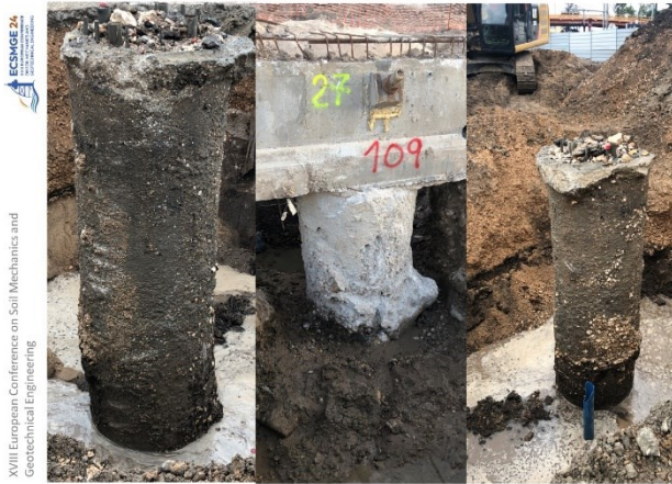
Figure 12 – Foundation piles anomalies.
