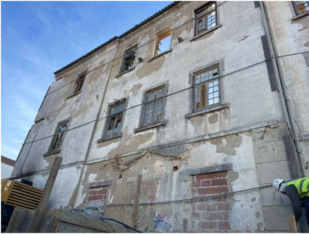
Figure 4 – Prior facade retention works, involving the installation of steel angles and steel tie rods per floor.
