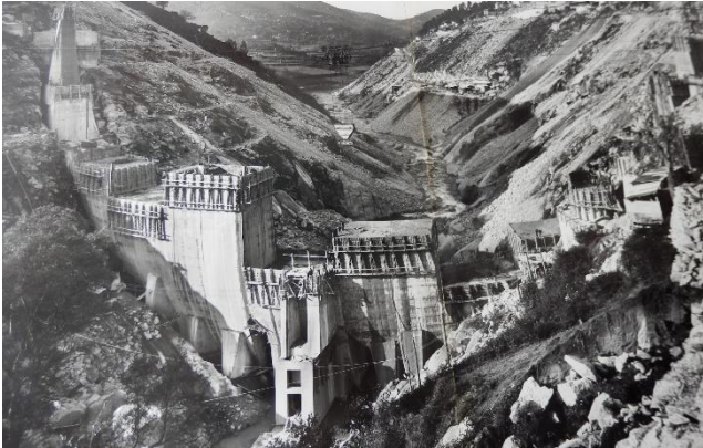
Figure 2. Construction of Caniçada dam reinforced concrete arch over granite bed rock (courtesy of Rodio).
